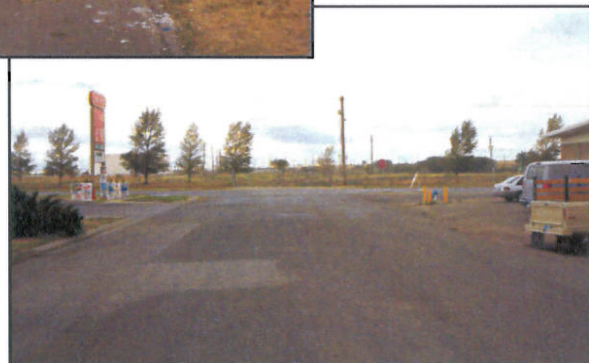
Many streets in the Corridor are in poor condition and do not have curbs or gutters.
